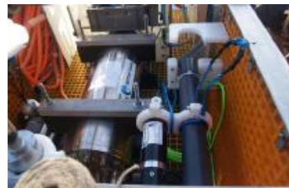
Junction Box installed on Deployment Rig (Credit: Venus)
